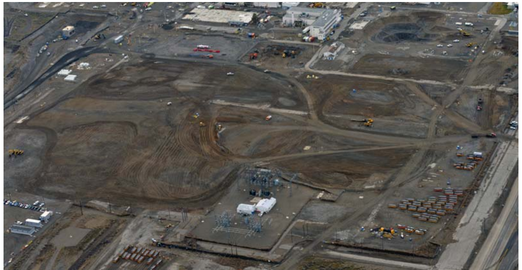
The north section of the 300 Area contained numerous highly contaminated facilities and waste sites.
