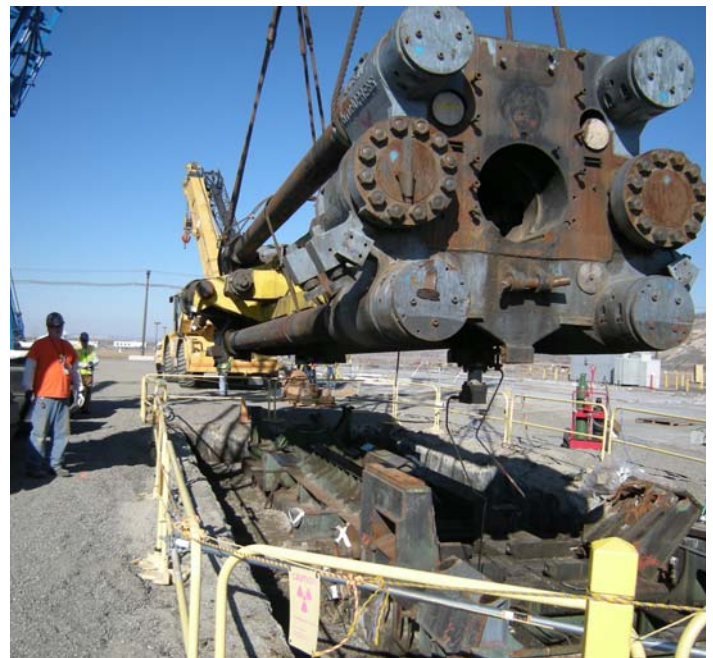
The Loewy Extrusion Press is removed from its foundation. The 2,750-ton press was housed in the 333 Building.
