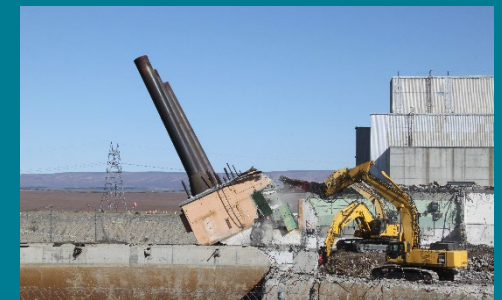
Demolition activities near the K East Reactor continue to change the Hanford skyline.
