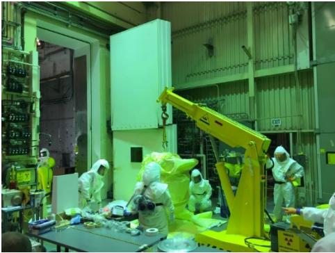
Workers safely remove waste from the airlock, an area adjacent to B Cell.
