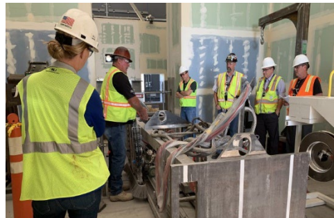
Workers installed and tested a saw at the mock-up that will soon be installed in B Cell to cut through the stainless steel liner and the concrete floor.
