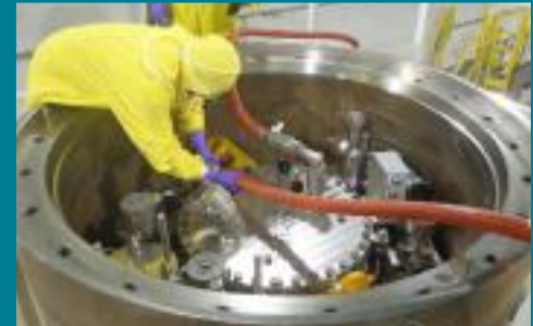
To prepare for receipt and storage of sludge containers, crews cleaned out large areas of the T Plant canyon (top), modified the cells beneath to accept the containers and performed extensive testing and training (above).
