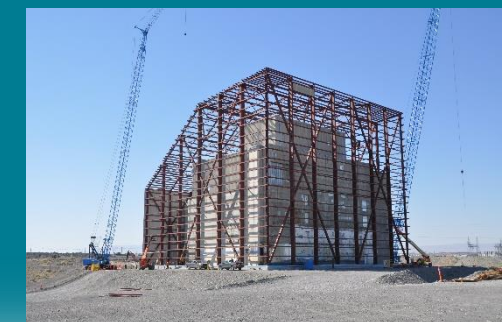
Work is nearly complete on a 123-foot-tall steel structure at the K East Reactor building. The structure, or cocoon, is designed to protect the building while radioactivity in the deactivated reactor core decays over the next several decades.
